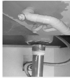
Water Supply Pipe Leakage/ Water Pipe Leakage
