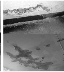
Roofs And Walls, Water Seepage In The Ground
