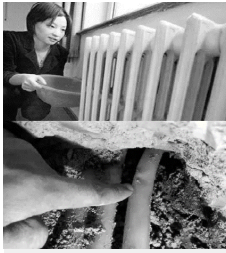
Heating Pipes/ Underfloor Heating Pipe Leaks
