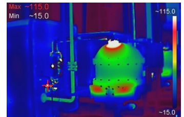
Check Mechanical Status
